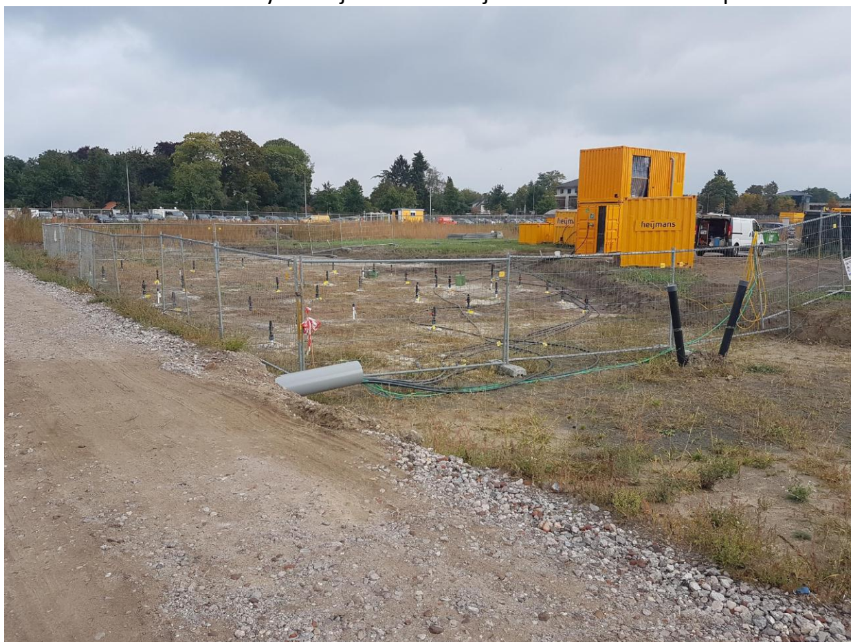
Overview injection filters in source zone
